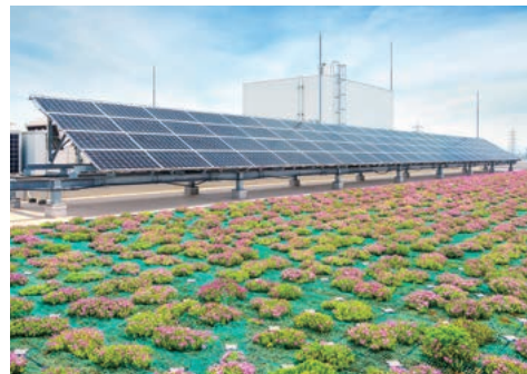
Solar panels on the Green Cycle factory rooftop
